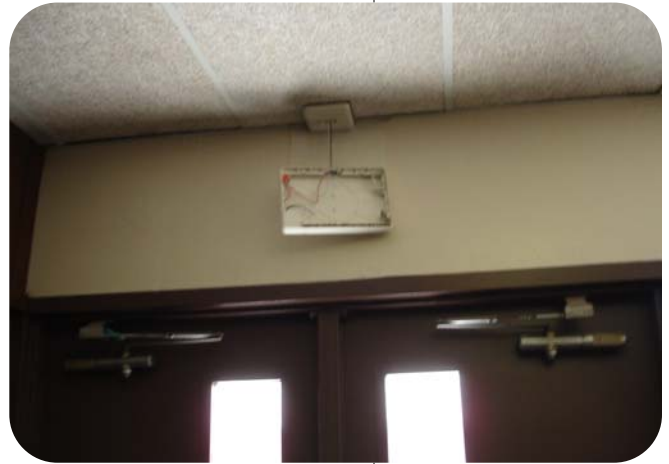
Damaged exit sign. Photo taken by Auditor General staff.
