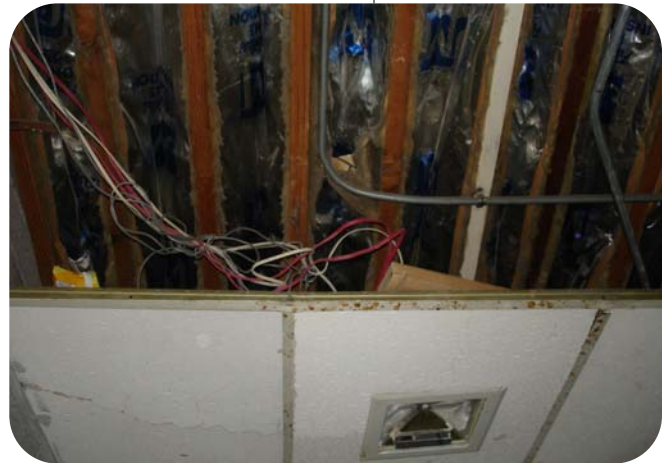
Missing ceiling tiles with exposed electrical wiring. Photo taken by Auditor General staff.
