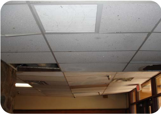
Damaged ceiling tiles. Photo taken by Auditor General staff.
