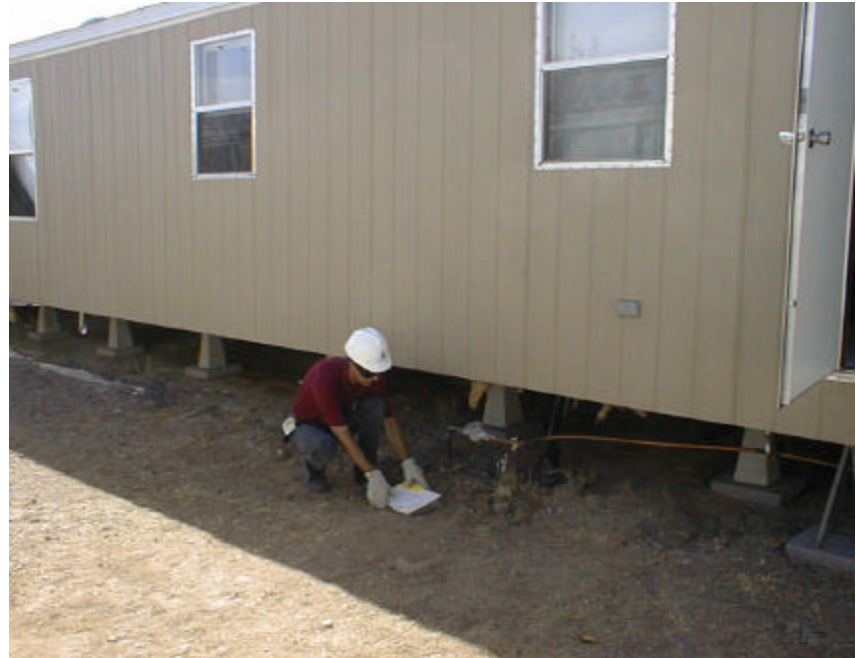
This Department employee is conducting an inspection to ensure the home is set properly on these piers.
