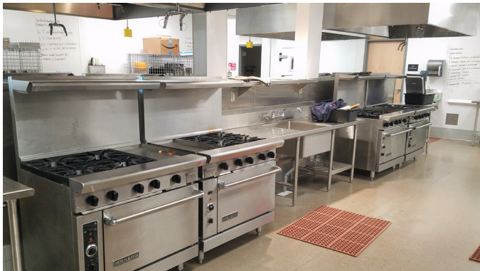
Kitchen with commercial equipment
