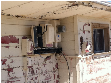
Exposed electrical wiring
