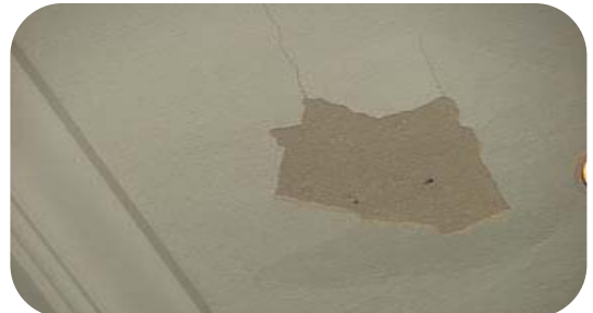
Photo 10: Water damage to a ceiling at UA's Centennial Hall
