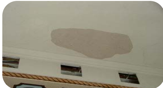
Photo 9: Water damage to a ceiling at UA's Centennial Hall
