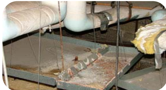
Photo 7: Deteriorated water lines at UA's Centennial Hall
