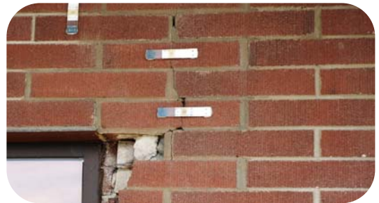
Photo 6: Cracked and crumbling exterior walls at NAU's Capital Assets Building
