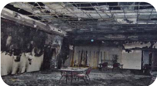
Photo 11: Damage caused by the November 2007 fire at ASU's Memorial Union
