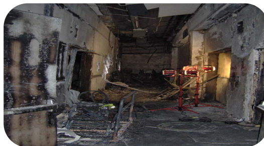
Photo 12: Damage caused by the November 2007 fire at ASU's Memorial Union
