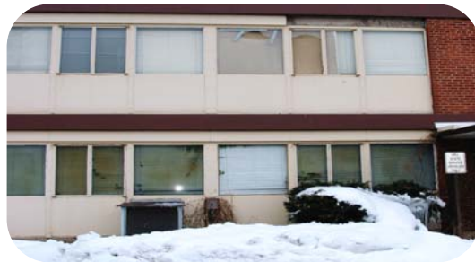
Photo 5: Broken and boarded-up windows at NAU's Babbitt Academic Annex
