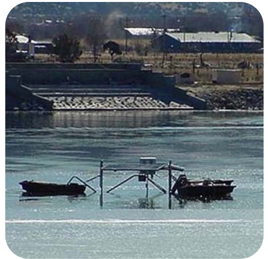
A solar powered aerator installed in the Town of Eagar's wastewater treatment system under the Hazard Mitigation Grant Program.
