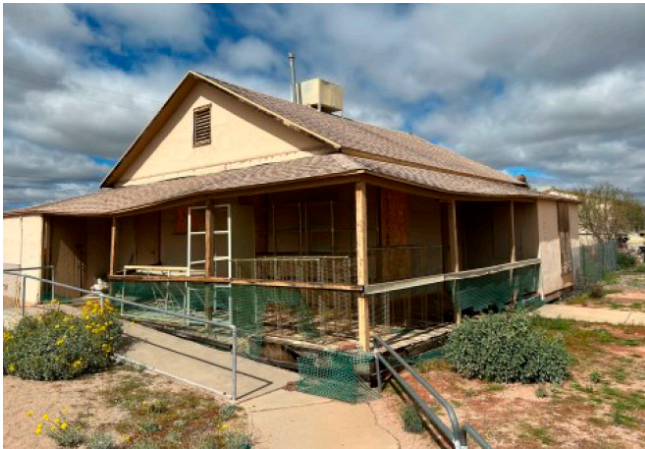
Photo 1 District building with potential structural deficiencies
