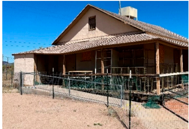
Photo 2 Metal fencing may be insufficient to restrict building access
