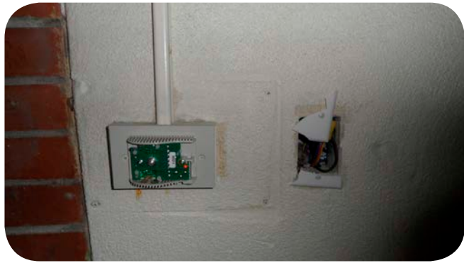
Photo 2: Exposed electrical wiring at high school
