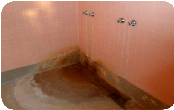
Water leak in middle school
