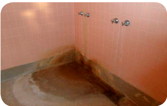
Photo 1: Water leak in middle school
