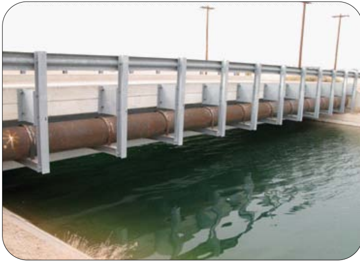
Photo 4: Section of Piping Connecting Water Systems in Eloy
