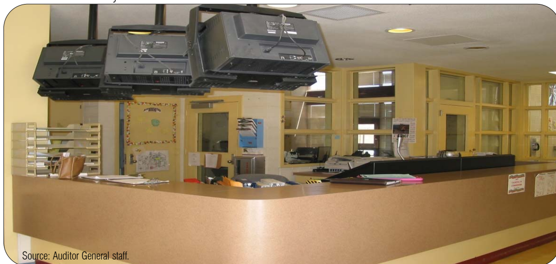
Photo 2: Mohave County Juvenile Detention Center Control Room
